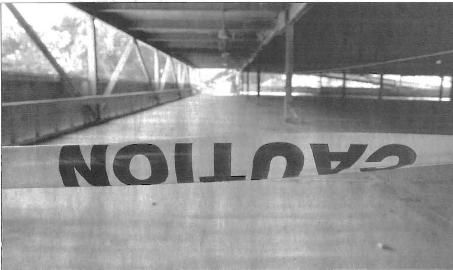
ABOVE: Garage N, located on West Drive located just north of the CCB, was closed to traffic at the end of May. The Office of Transportation and Parking Services cited the garage's deteriorating condition as the reason for its closing.
